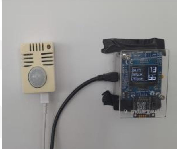
BatSense and neOSensor devices mounted in wall of the HW laboratory at CEDINT-UPM
